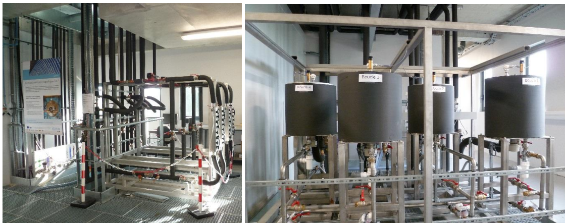
Figure 1 : Alphéo II : on the left : view of four distribution networks; on the right :view of four heaters
